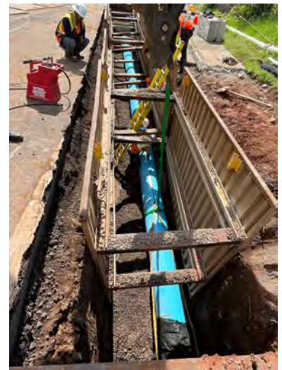
Utilities privatization contractor repairs sewer line in Oahu, Hawaii. Photo credit: Aqua Engineers
